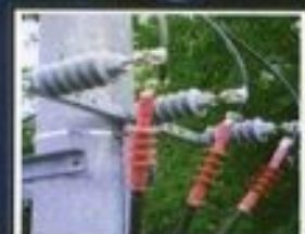
Outdoor Surge Arrestor
